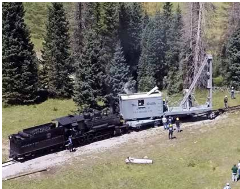
Top: There are 7 pile trestles on the OC&E's Sycan Branch; this is the largest one, both in length and height. As they were built in the 1920's they probably needed most of the exposed wood replaced at least once during that time. Bottom: On Sunday, August 28, 2016, the Cumbres and Toltec Scenic Railroad provided a demonstration of Pile Driver #OB on the tail of the wye at Cumbres Pass. The Durango Railroad Historical Society restored D&RG #315, a 2-8-0 built in 1895 and it provided the power for the pile driver, and members of the Friends of the Cumbres and Toltec Scenic Railroad operated OB. Drone photo by Roger Hogan
